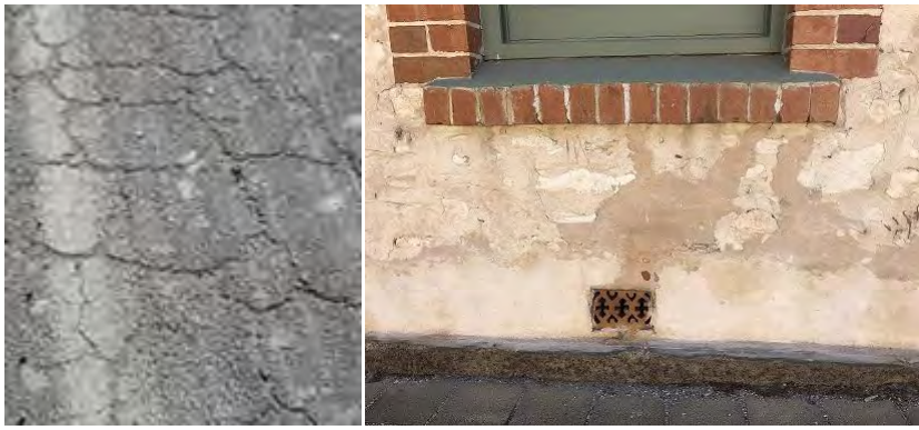
Salinity affected road and building foundation. Photo credit: NSW Government Repairs as a result of rising salt damp at Tintinara CWA Building
