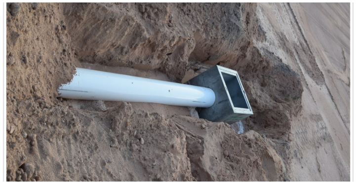
Concrete sump and outlet.
